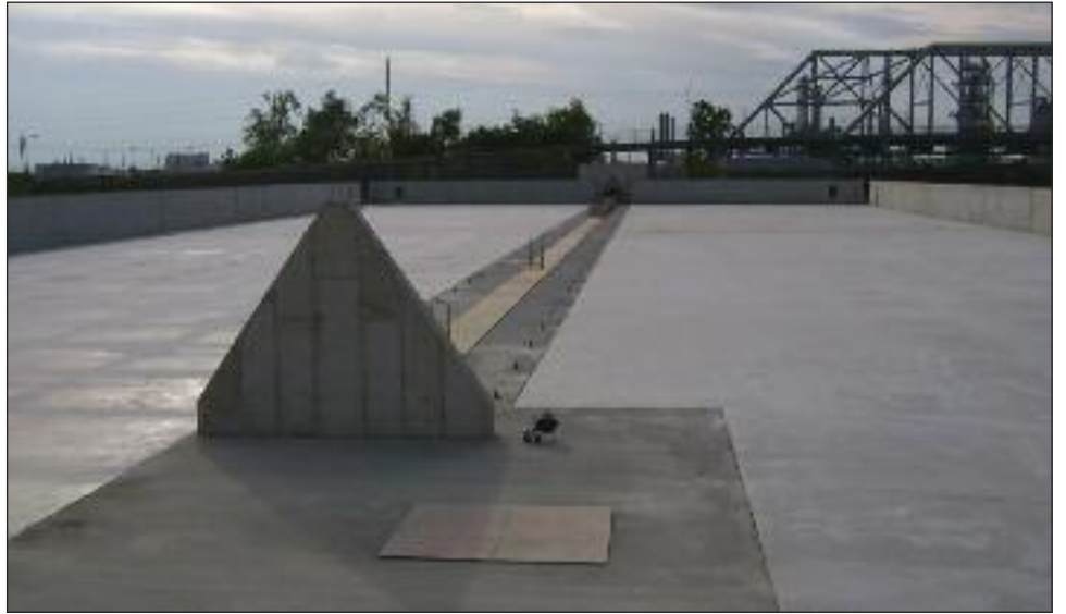
Lima Energy fuel storage building under construction. (Photo courtesy of Global Energy, Inc.)
